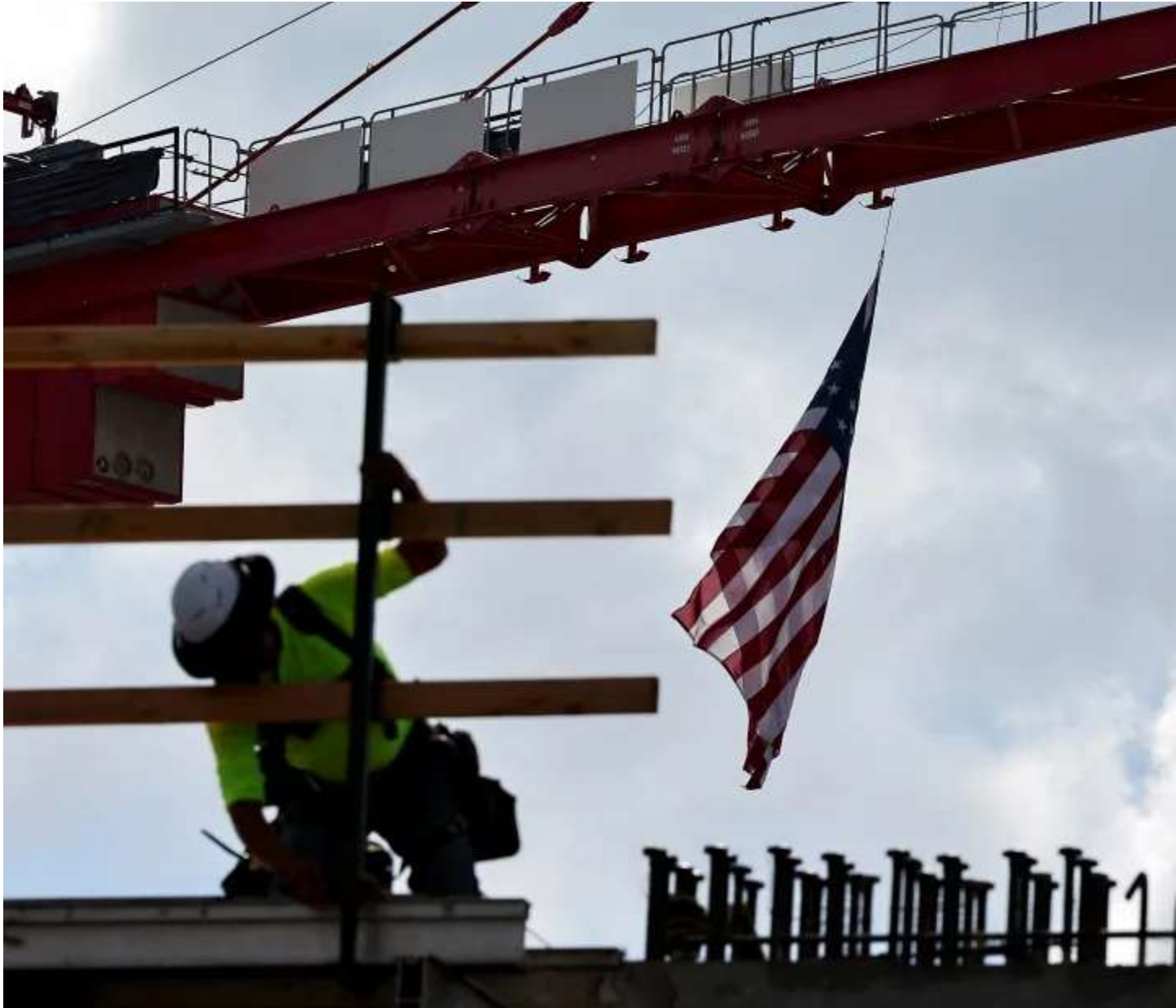
An American flag flies from a crane as a construction worker helps build a mixed-use apartment complex on Jan. 25, 2024, in Los Angeles, California. (Mario Tama/Getty Images) (Mario Tama via Getty Images)
